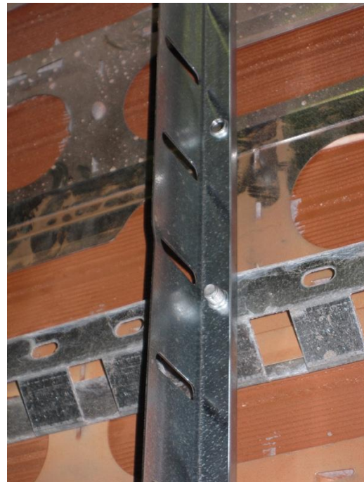
Photo 4. Start of failure with buckling of web of vertical rail.
